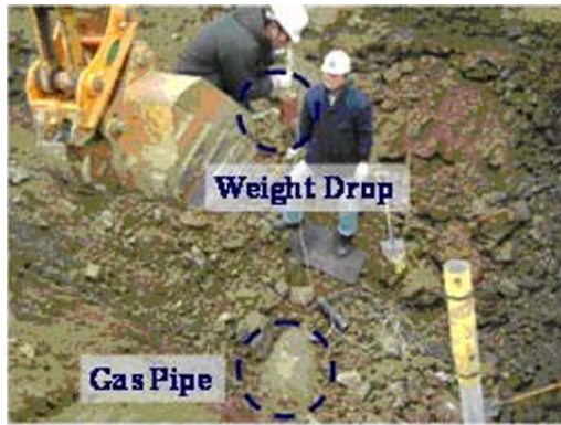
Fig. 15. Photograph of the impact process used to measure the wave propagation properties of a buried gas duct.
